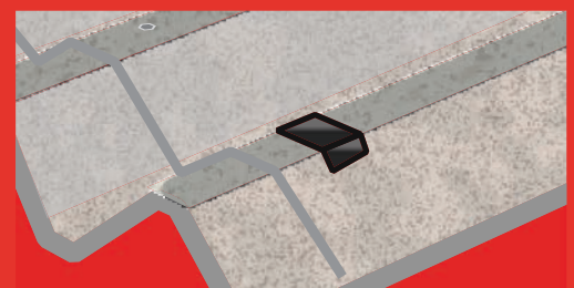
Liquid Rubber High Build applied to the exposed bolt head and the surrounding area.
